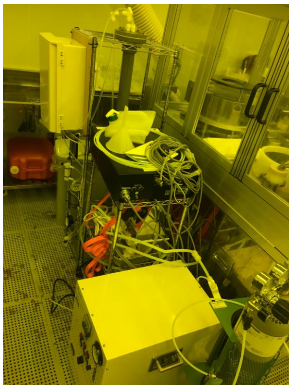
Fig1. Photoresist Removal Equipment
